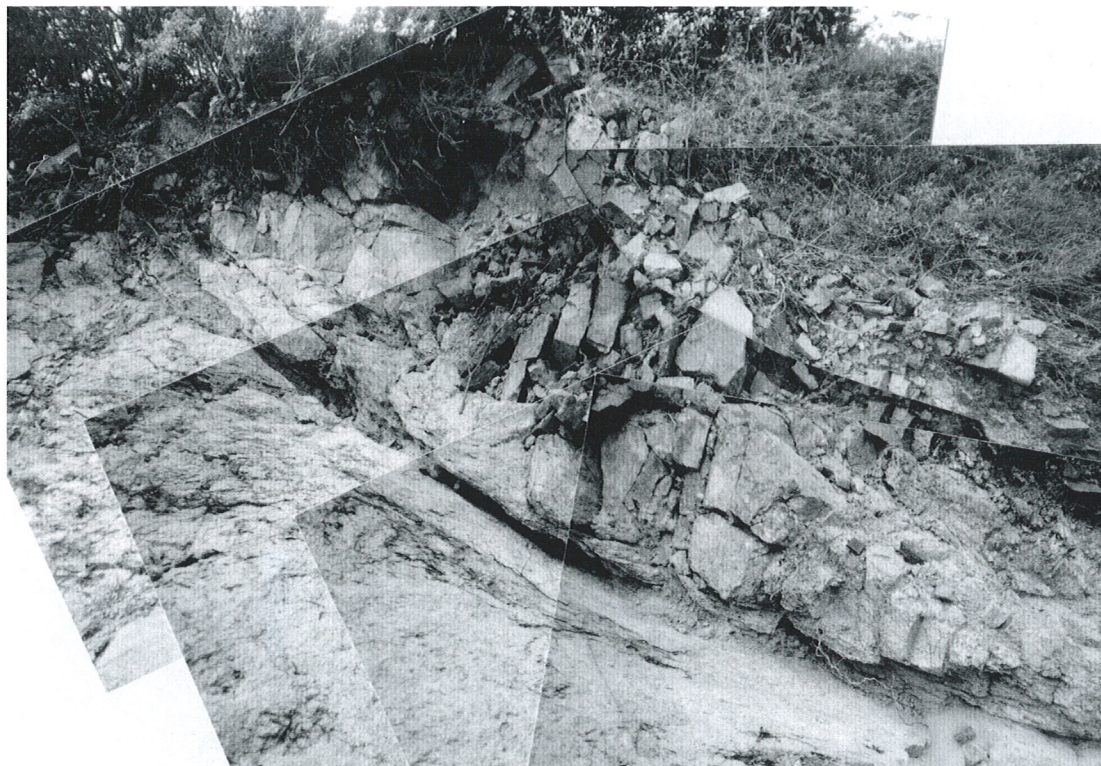
Plate 4 Landslide 1, Tsing Shan. Basal release surface controlled by sheeting joint dipping 44-60°/166-198°. Note the preferential weathering along the joint surface and dilation of overlying rockmass.
